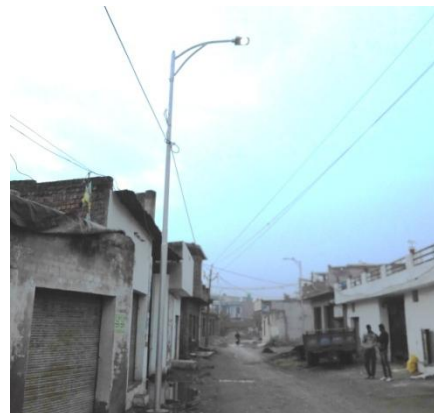
LED light installed in Ward 26
