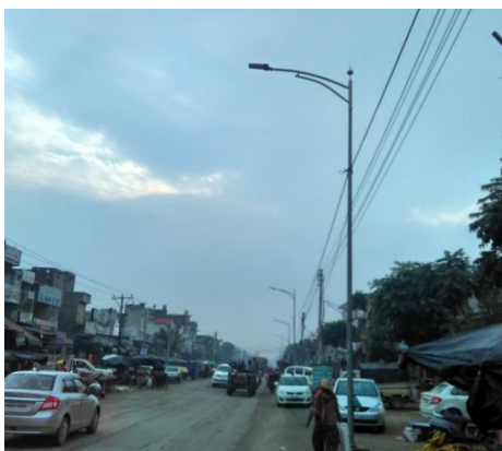
LED light installed along GT Road
